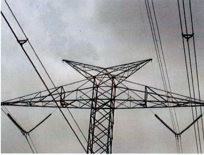
Picture caption: The two thin wires, suspended from the top of the tower, between the more visible bundled lines, are the static shield wires.
