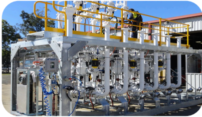
Tanker Loading Gantries
