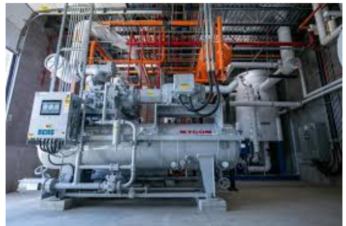
Ammonia Refrigeration System
