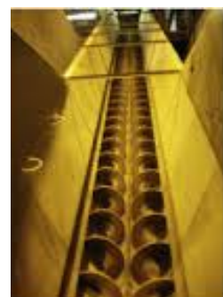
Screw Conveyor System
