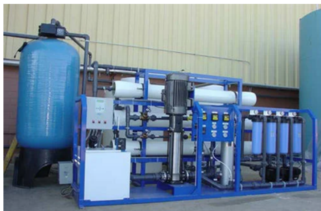
Reverse Osmosis System
