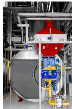
Air Preheat System
