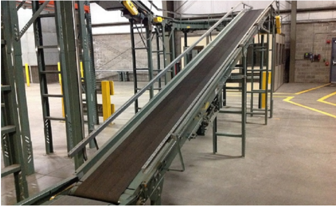
Belt Conveyor system
