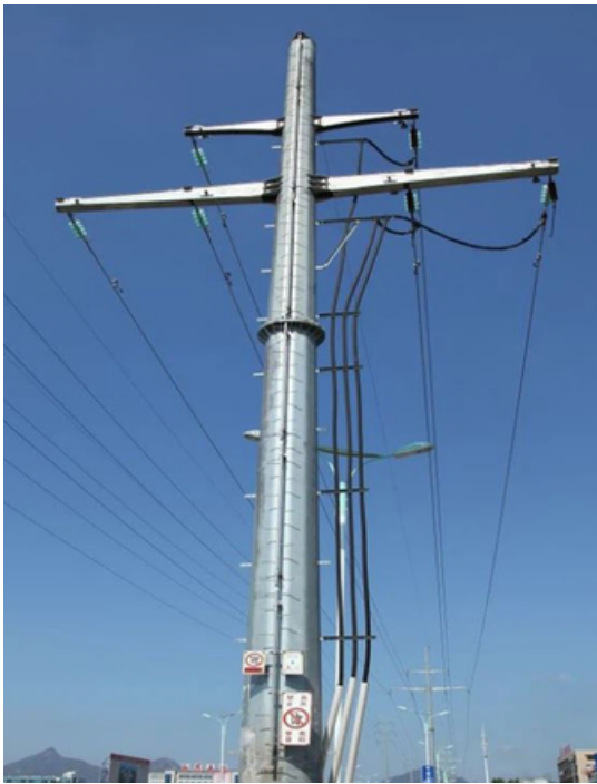
Low Voltage /High Voltage Transmission Pole
