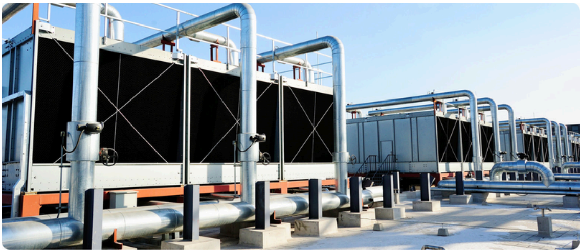
Heat Exchanger for Cooling tower
