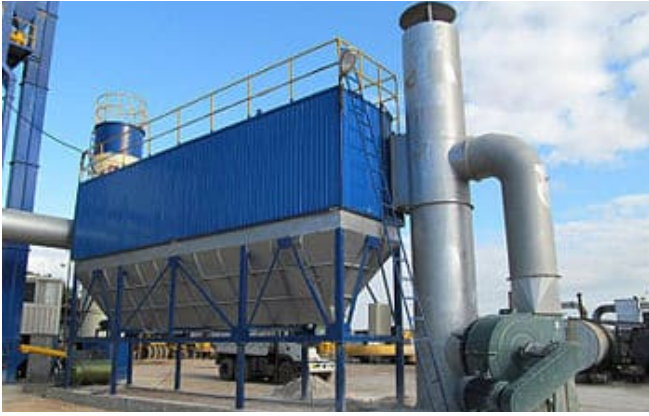
Dry Dedusting System
