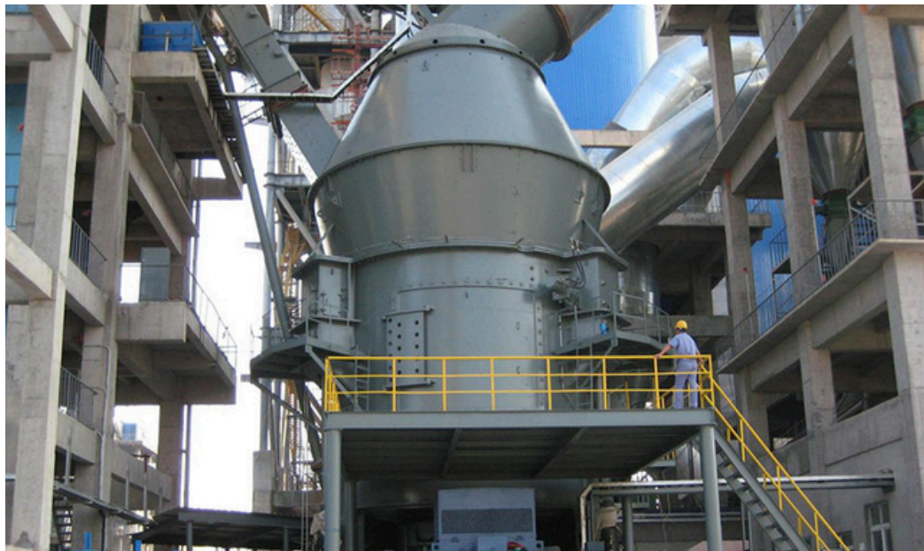
Cement Clinker Milling Plant
