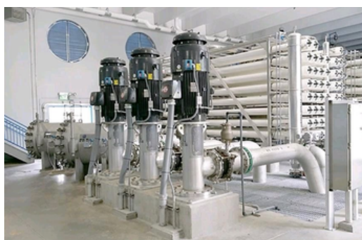
Sea Water Desalination System
