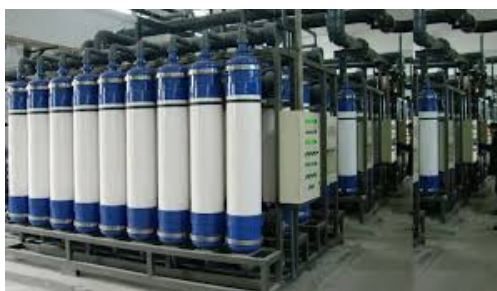
Ultra Filtration System
