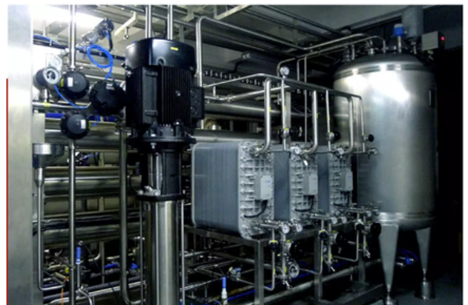
Electro Deionisation/demineralisation system
