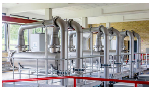
UV disinfection System
