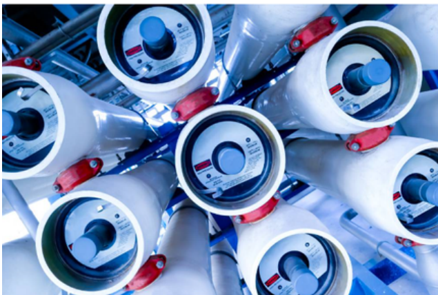
Nano Filtration Unit
