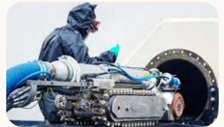
Tank cleaning equipment
