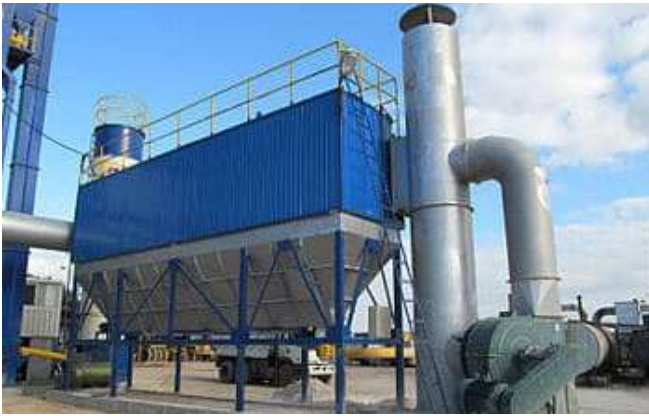
Dry Dedusting System
