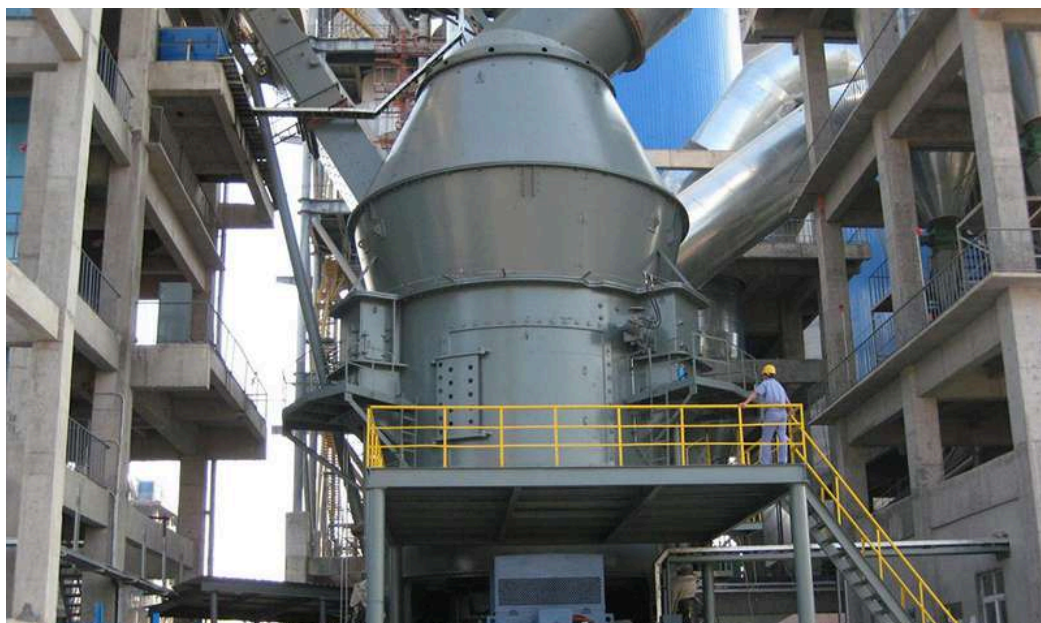
Cement Clinker Milling Plant
