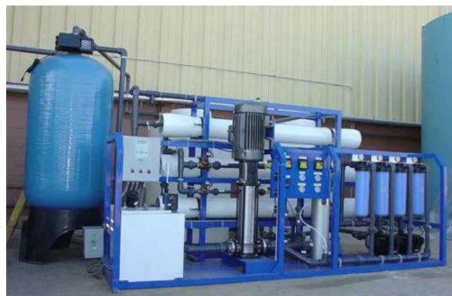
Reverse Osmosis System
