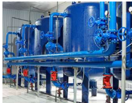
Zero Liquid Discharge system
