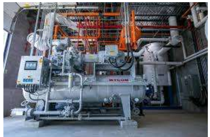
Ammonia Refrigeration System
