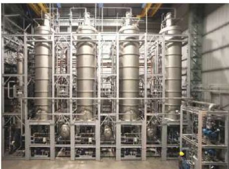
Shortpath Distillation Unit
