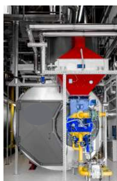
Air Preheat System
