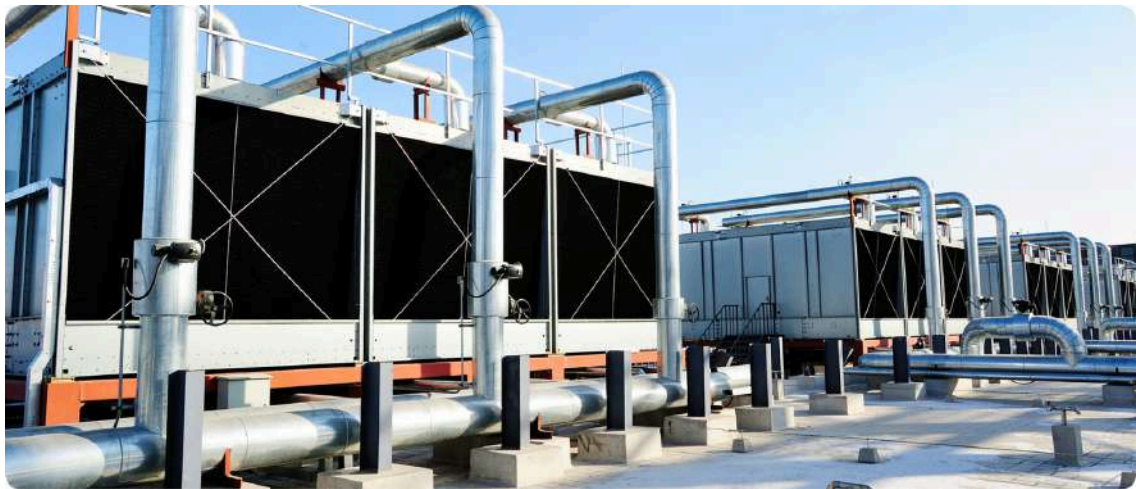
Heat Exchanger for Cooling tower
