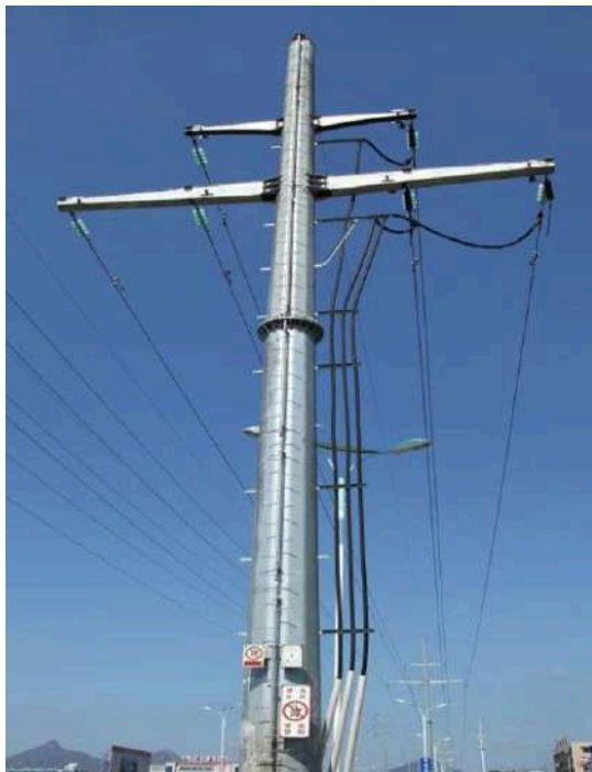
Low Voltage /High Voltage Transmission Pole
