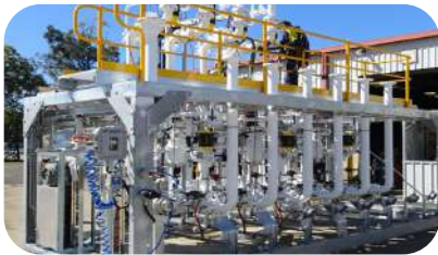
Tanker Loading Gantries
