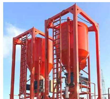
Cement Surge Tank
