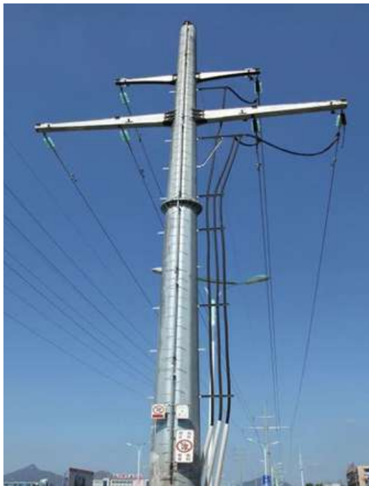
Low Voltage /High Voltage Transmission Pole
