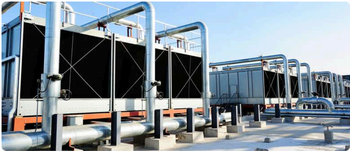
Heat Exchanger for Cooling tower
