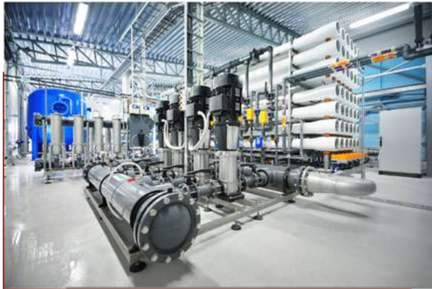
Sea Water Reverse Osmosis System
