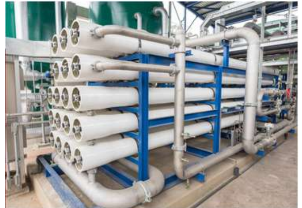
Brackish Water Reverse osmosis system
