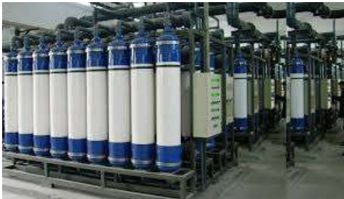
Ultra Filtration System
