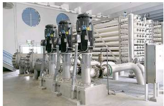
Sea Water Desalination System
