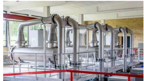
UV disinfection System
