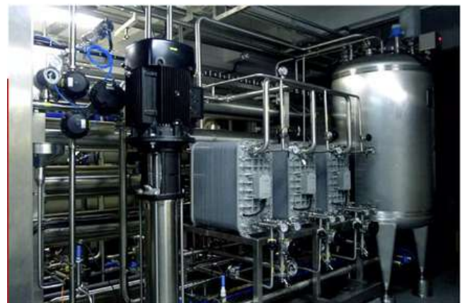
Electro Deionisation/demineralisation system
